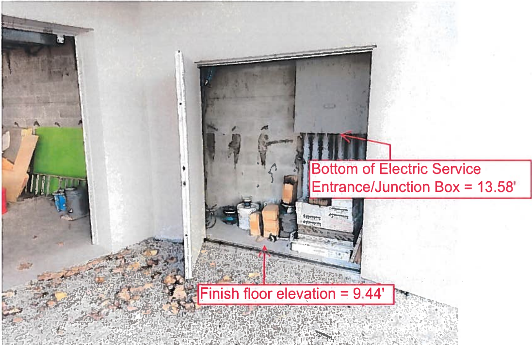
(01/22/2019) Electric Service Panel at ground level
