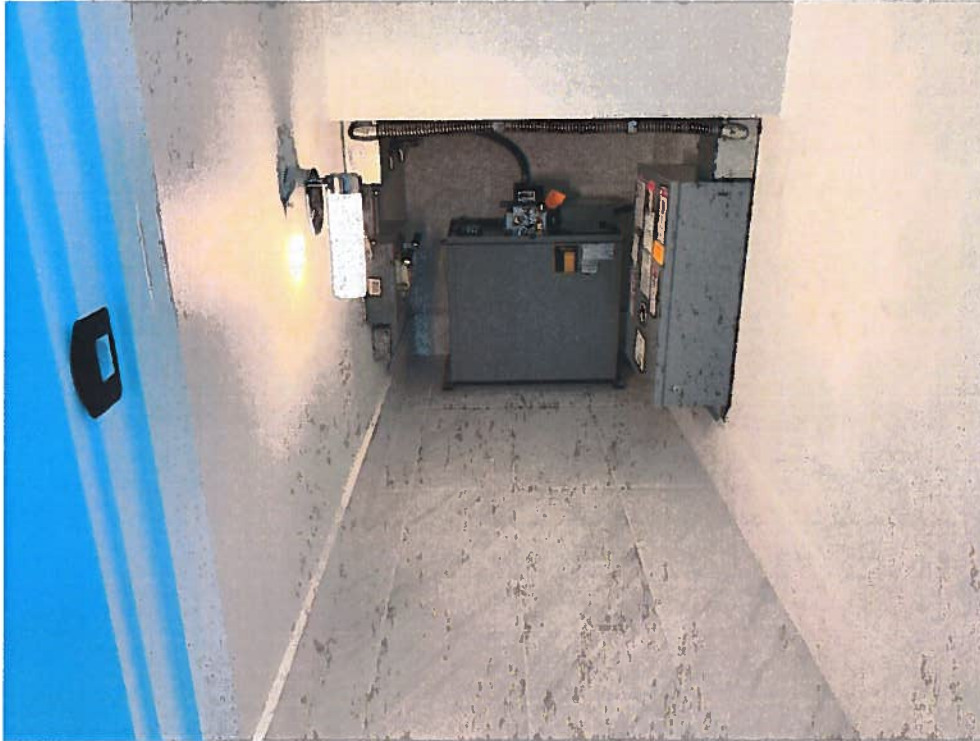
(05/06/2021) Elevator Equipment on 1 st Living Area Finish Floor
