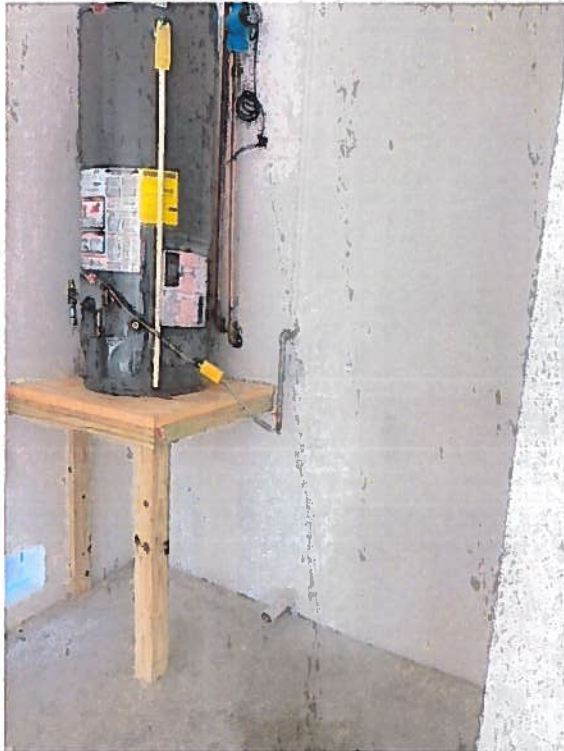
(05/06/2021) Elevated Hot Water Heater in Garage Area
