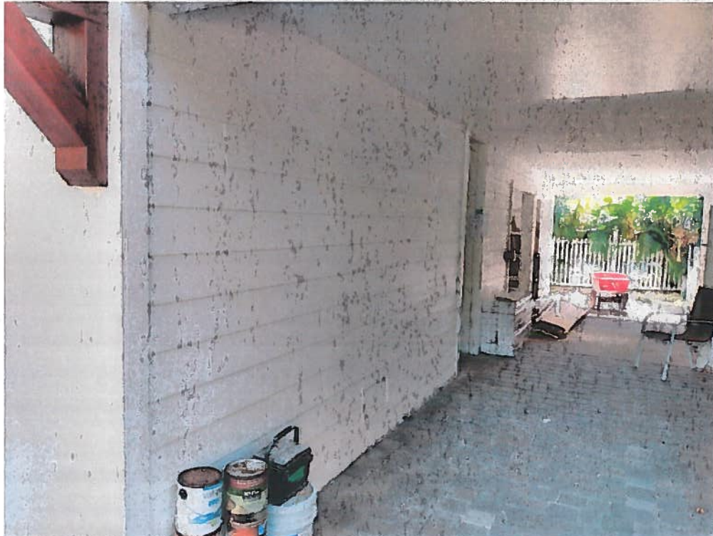
(10/11/2021) Right Side of Storage & Entry Enclosure with Smart Vents & Parking
