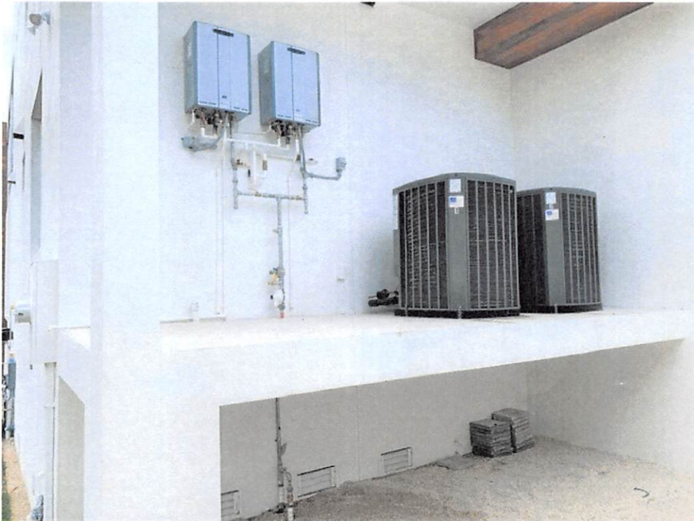
(10/23/2021) Elevated AC Units and Tankless Water Heaters
