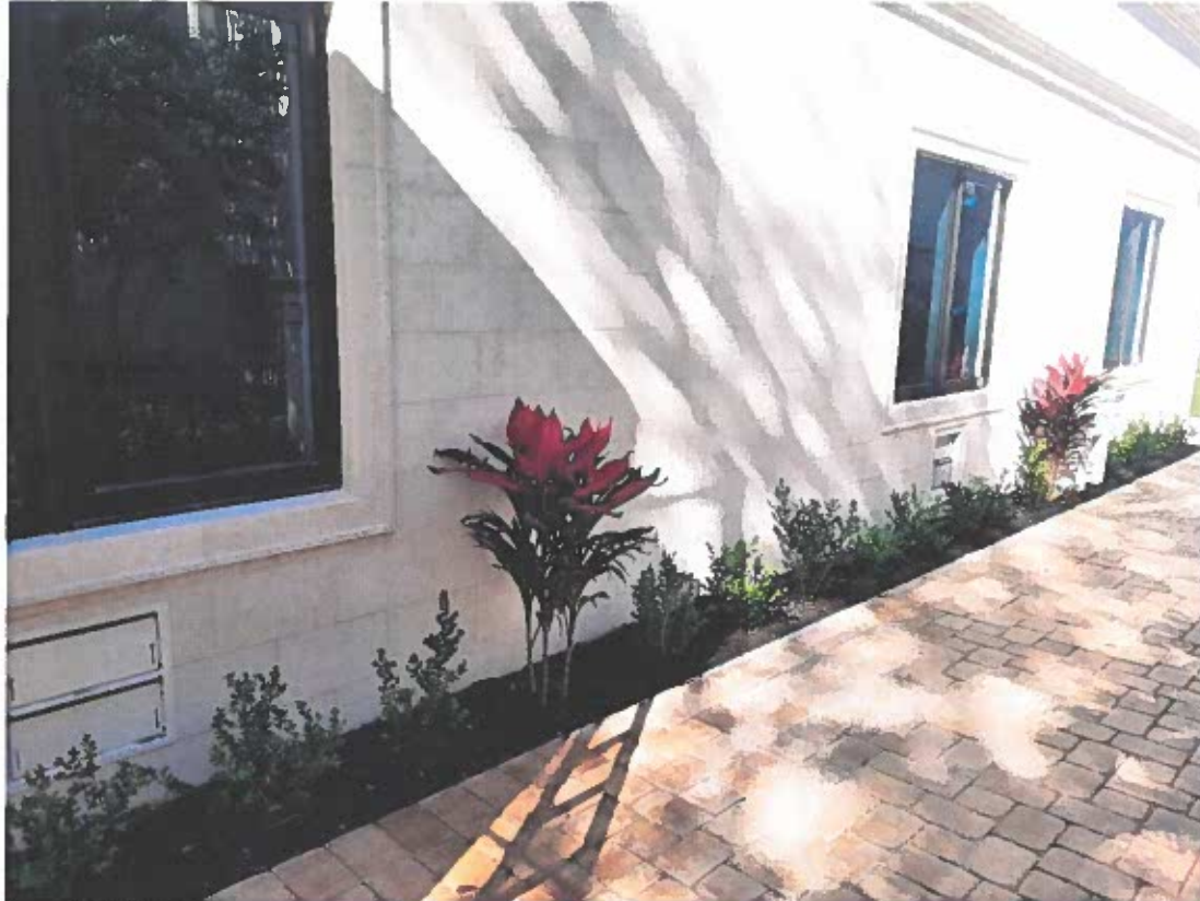
(02/13/2023) 3 Double Smart Vent Model #1540-521 on Right Side-Rear Portion of Storage 1 & Storage 3
