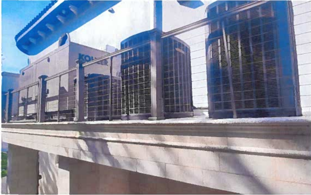
(11/17/2022) Elevated AC Units and Generator
