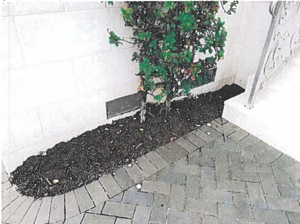
(12/30/2022) 2 Smart Vents Model #1540-520 on Right Side Garage Wall
