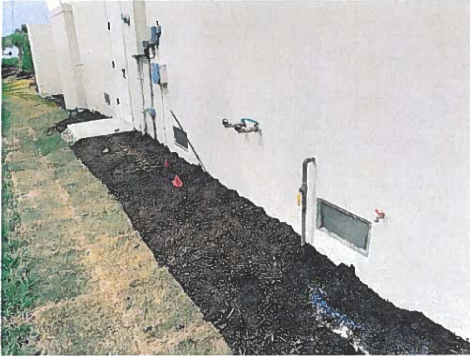
(12/30/2022) 3 Smart Vents Model #1540-520 on Left Side Garage Wall
