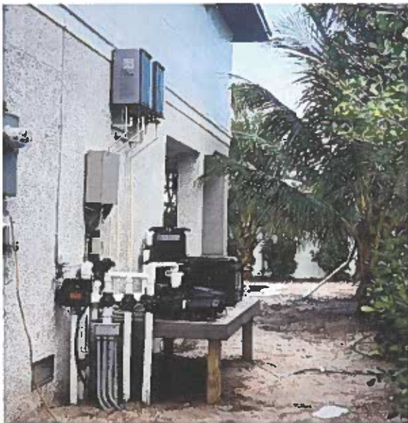
SIDE / WATER HEATER
