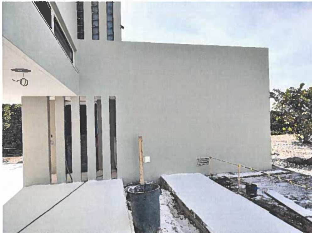
(05/05/2023) West Side of South Structure Enclosure #2 With 1 Smart Vent
