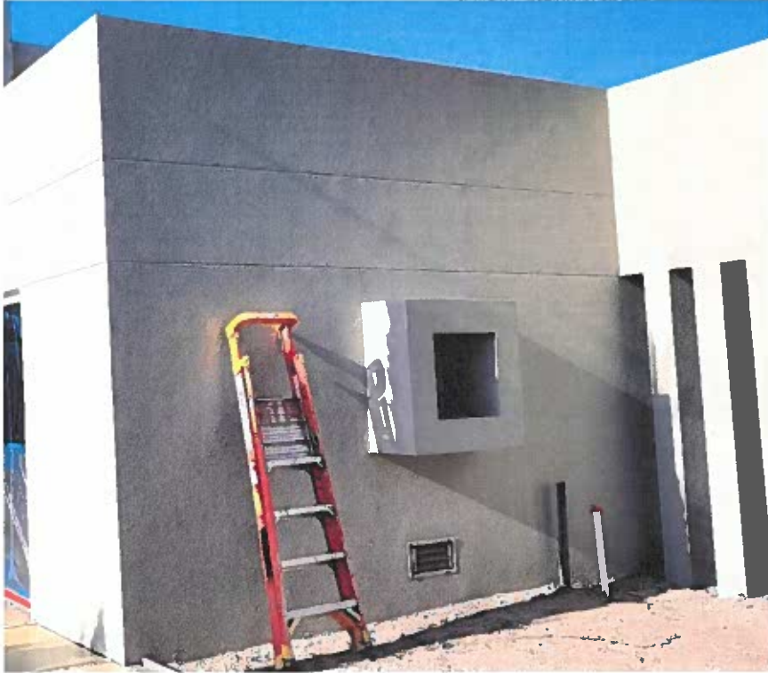
(05/05/2023) North Side of North Structure Enclosure #1 with 1 Smart Vent
