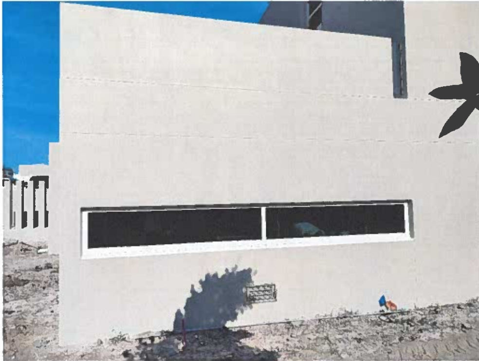
(05/05/2023) East Side of the South Structure Enclosure #2 With 1 Smart Vent
