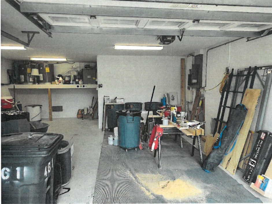
(12/13/2023) Bottom of Electric Panel Box= 10.1'. Platform for AC, Hotwater Heater & Elevator Equipment Located in Garage= 10.4'.
