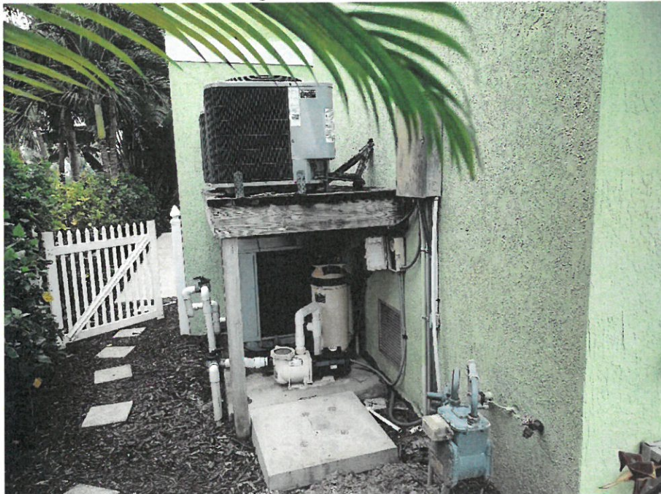
(12/13/2023) Platform for AC=10.5', Outside Back Right Side of Structure. 1 Non-Engineered Vent in Right Side of Storage.
