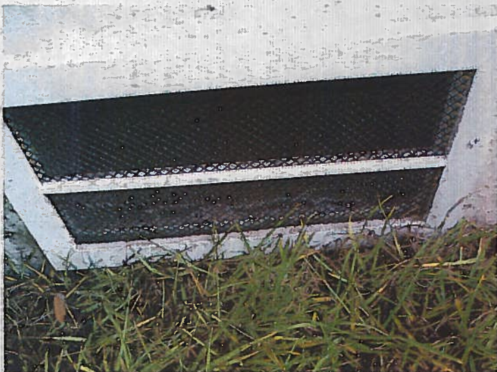
Typical Flow Through on Garage Walls Photographs Date Taken 5/18/2016
