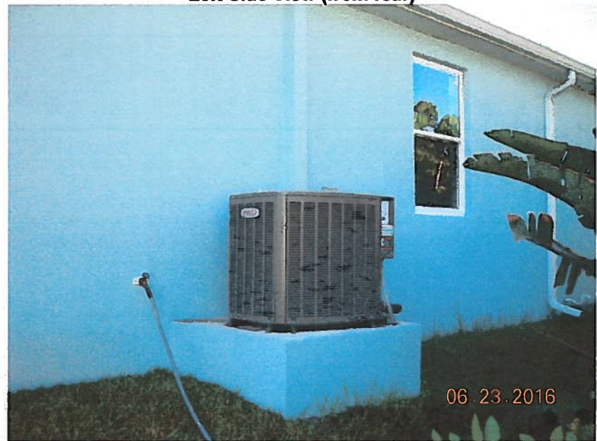
Elevated A/C pad
